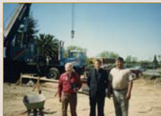
As construction commences, three key people are regularly on the scene. Jim Hiltz (the Parish's construction superintendent), Father Vereker, and Martin Rodriguez
