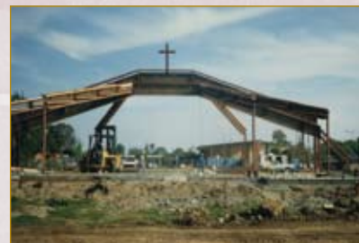
By April of 1988, the frame for the church began to appear, as girders were lifted into place
